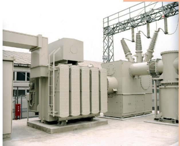
3φ 60Hz 75.25/6.6kV 7,500kVA
