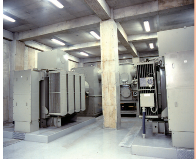
3φ 50Hz 64.5/6.6kV 3,000kVA
