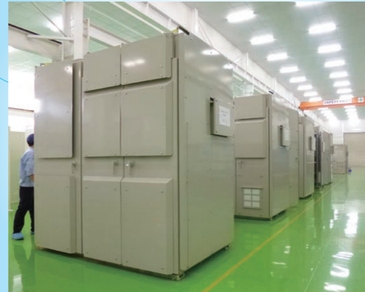
Power conditioner enclosures
