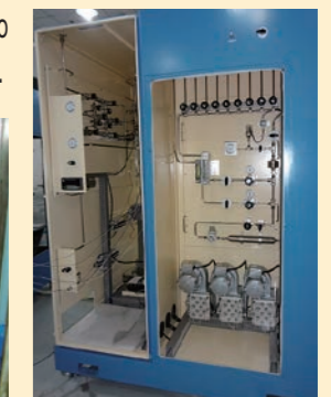
Gas flow rate control equipment
