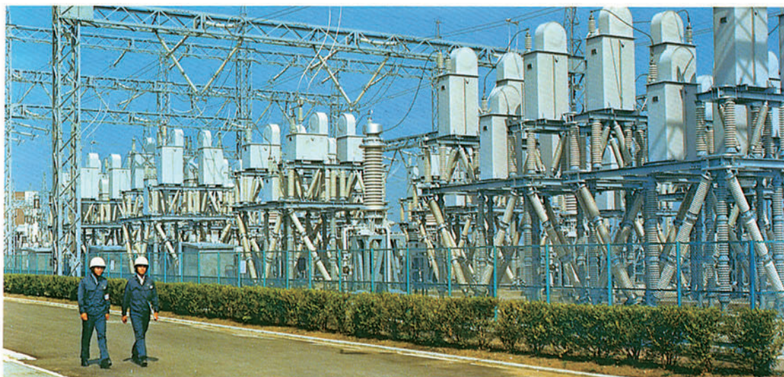
275 kV AC harmonic filter equipment 132 Mvar
