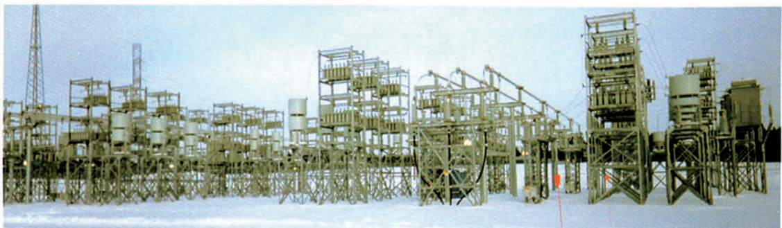
69 kV AC filter equipment 3\phi 60 Hz 176 Mvar
