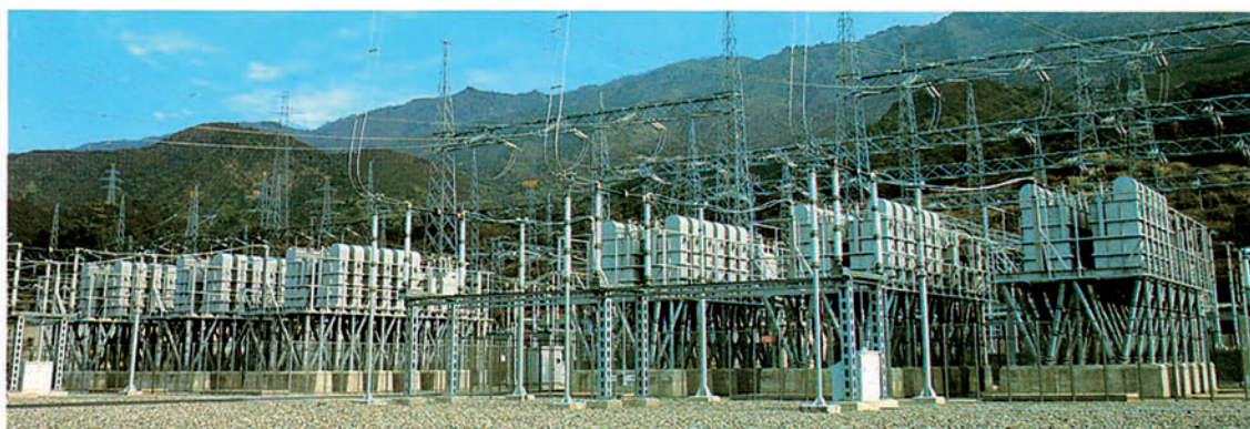
275 kV Series capacitor banks 20.4 \Omega 49.6 Mvar \times 2
