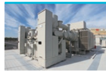
77kV Extra-high Voltage Substation Equipment
