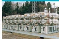
154kV Gas Insulated Switchgear
