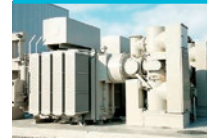
66/77kV Oil Filled Transformer
