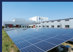
Captive Consumption Photovoltaic System
