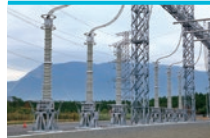
550kV Capacitor Voltage Transformer
