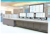
Supervisory Control System for Waterworks
