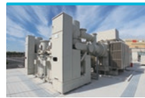
77kV Extra-high Voltage Substation Equipment
