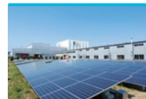
Captive Consumption Photovoltaic System
