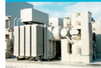
66/77kV Oil Filled Transformer
