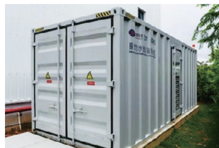
Membrane water treatment equipment
