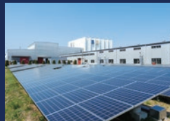
Captive Consumption Photovoltaic System
