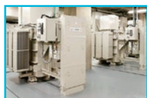
22/33kV Spot Network Substation Equipment
