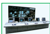
Supervisory Control System for Waterworks
