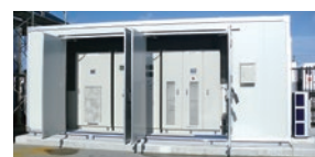
Storage Battery System
