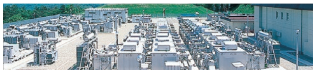
66/77kV Harmonic Filter Equipment
