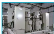
66/77kV Gas Insulated Switchgear (Indoor Type)
