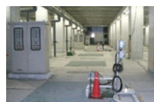
An installed ammonia nitrogen monitor
