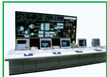
Supervisory Control System for Waterworks
