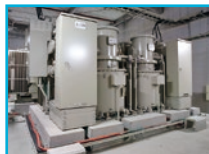
66/77kV Gas Insulated Switchgear (indoor type)
