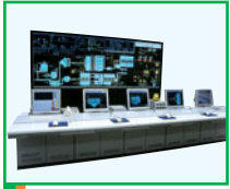
Supervisory Control System for Waterworks
