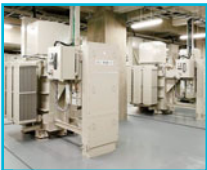
22/33kV Spot Network Substation Equipment
